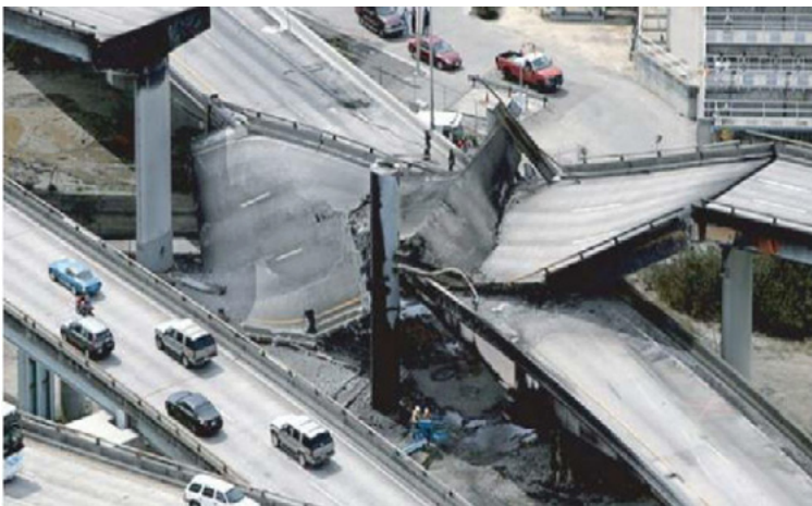
Figure 5. The I-80/880 Highway bridge collapse, MacArthur Maze Interchange, Source: New York Times, 2007 [31]
