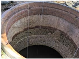
Cover Frame Corrosion
