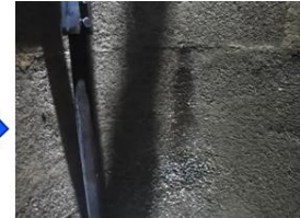
Concrete Wall Leaking
