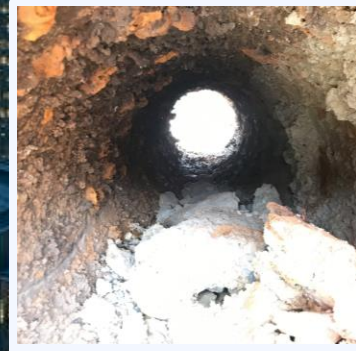
Internal corrosion / tuberculation in unlined sections
