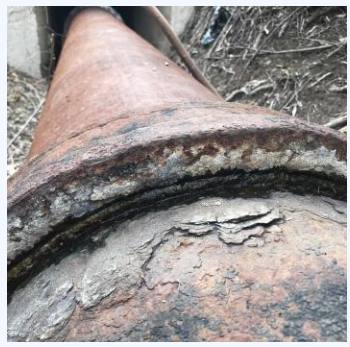
Movement of joints due to varying ground conditions leading to leakage
