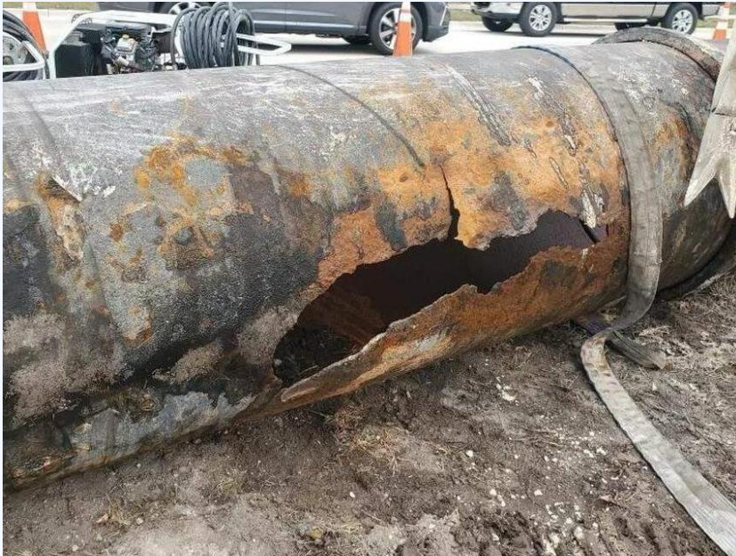
Florida Keys (USA) – Water Main Burst (2023)
