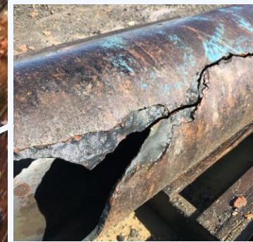
Catastrophic failure due to overloading (transients, traffic, etc)
