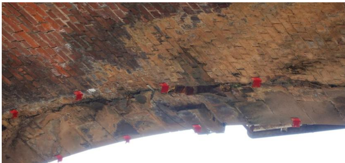
Figure 13. Longitudinal crack between the spandrel wall and the arch barrel
