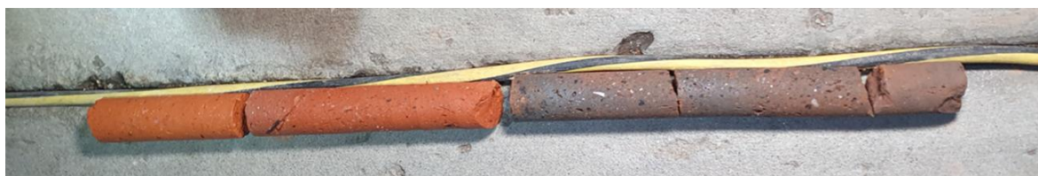
Figure 2. Core 4 through bridge abutment – ‘Void’ filled with mass concrete / grout (shown on the right-hand side)
