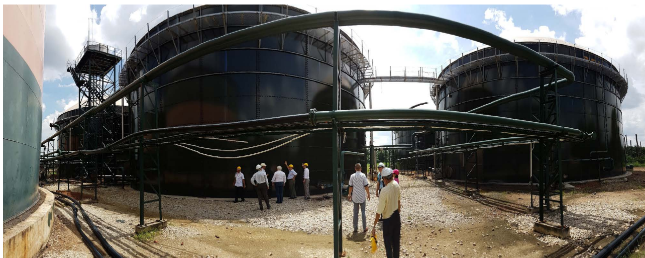
Figure 3: CSTR AD Tanks
