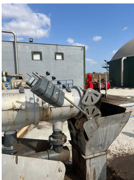
Figure 8: Post Treatment Sludge Dewatering
