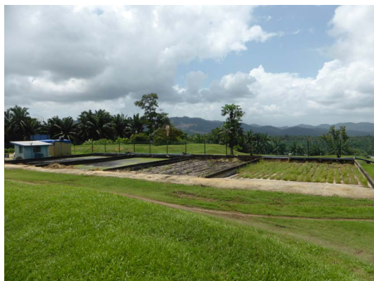
Figure 5: Sludge drying bed
