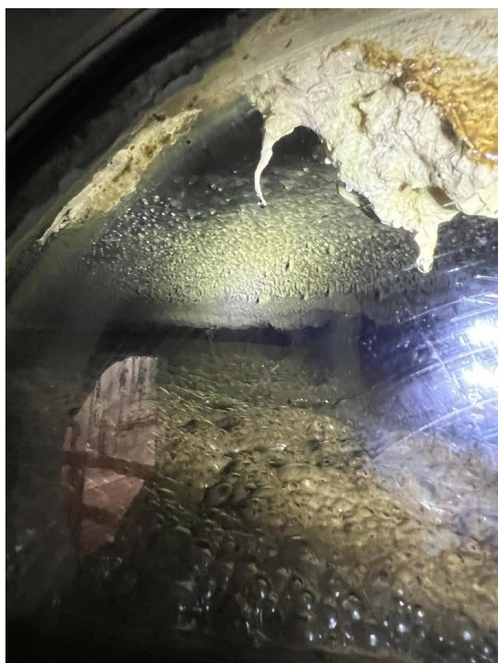
Figure 4: View inside digester
